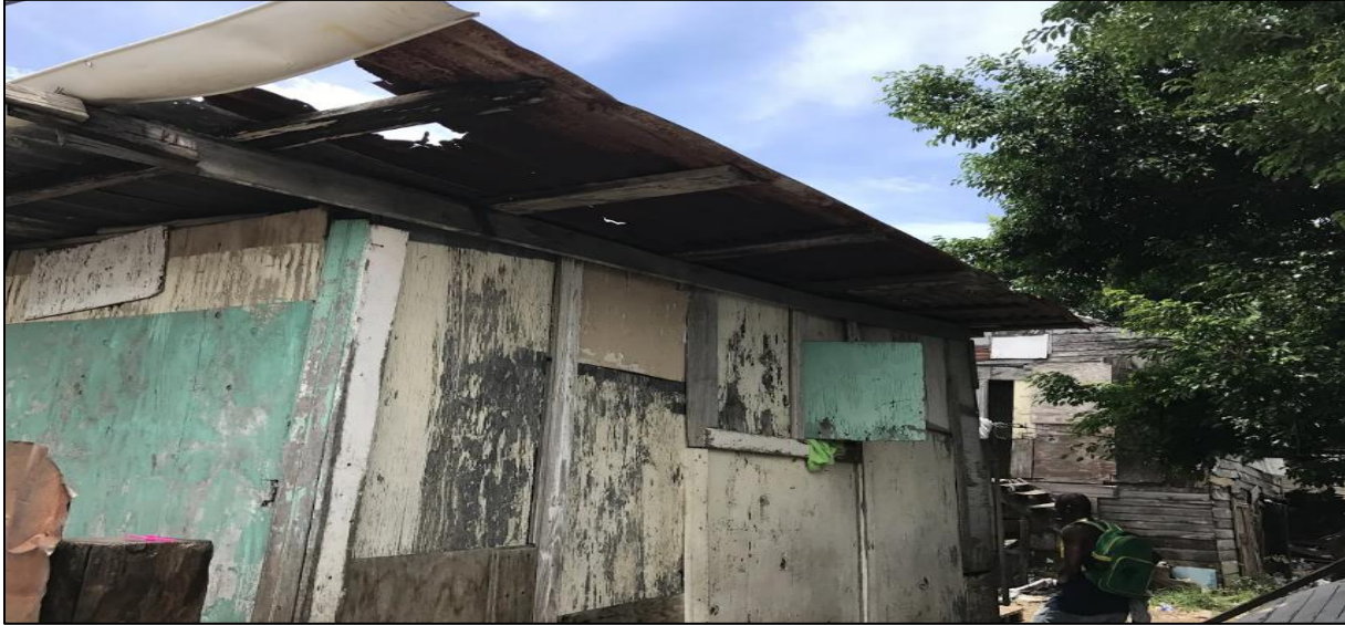
Image 9: Between Canals 187B is an example of an improvised structure. Wood, plywood, and metal make this structure.
