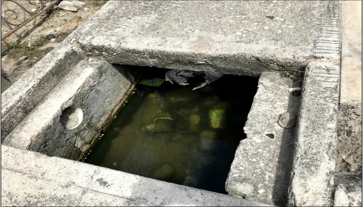
Image 6: (N 17.49710 W 088.19930) An open drain near Between Canals plot 1 is a possible breeding site for mosquitoes.
